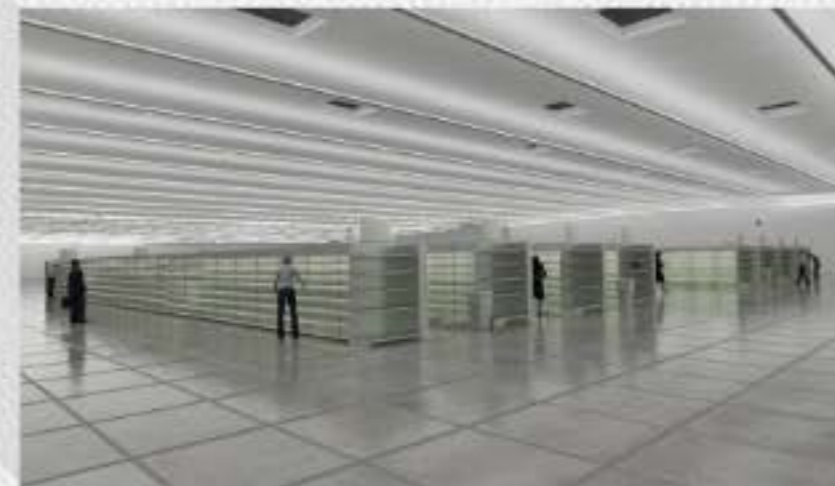
Ceiling Lighting at 25% Shelf Lighting at 0.25W/ft
